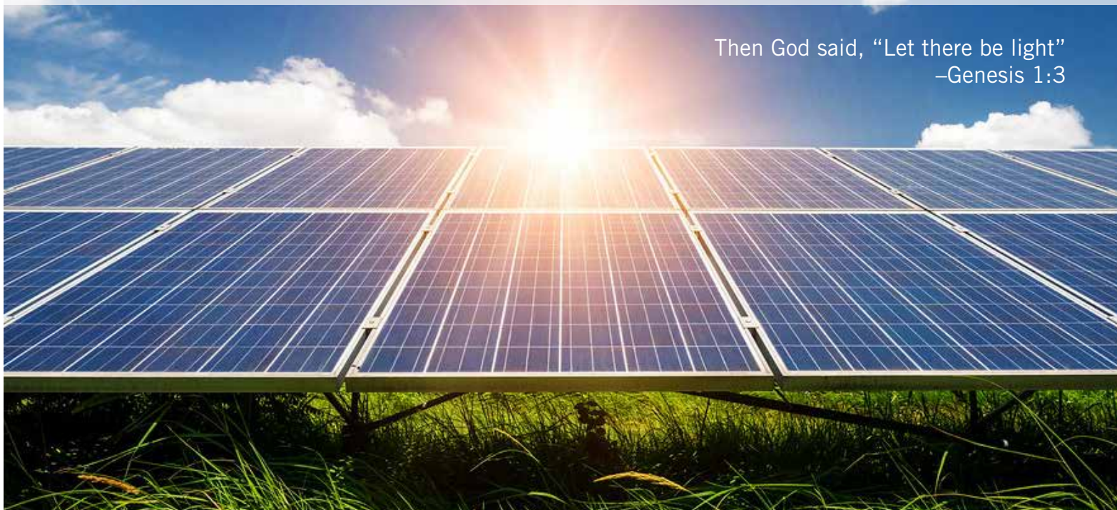
MG&E Middleton Airport Solar Array
