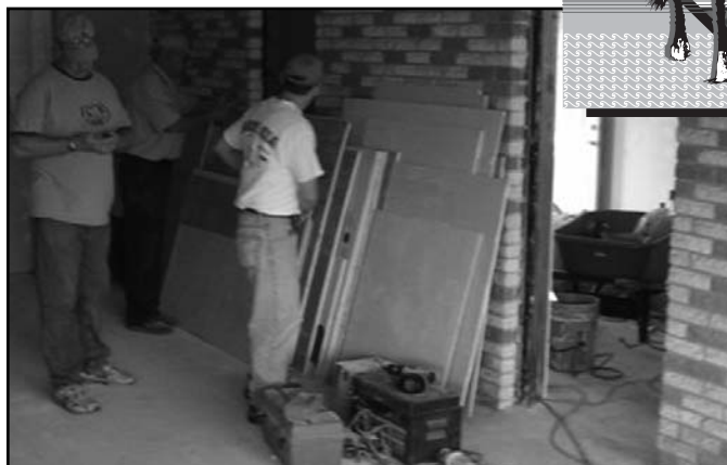
Bethel volunteers helped with drywall, painting, refinishing floors and carpentry work as part of the mission trip to New Orleans earlier this year. Funding from the Bethel Endowment Foundation helps support mission projects locally and around the world.
